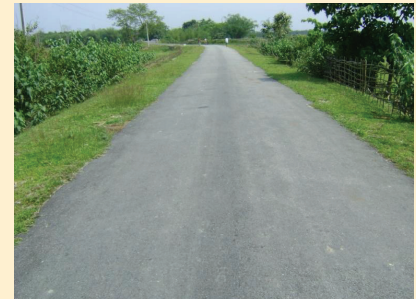
Condition of the road after 2 year
