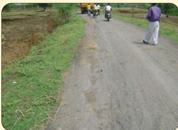
Initiation of distress at Control section after 26 Months (2009)
