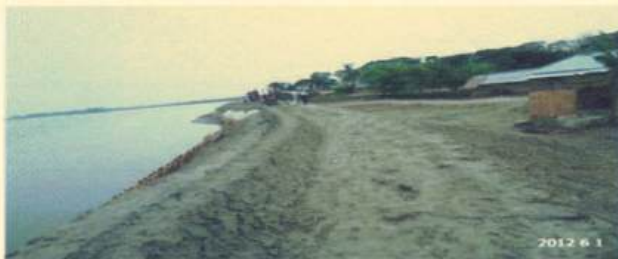
Fig: Pre-work Condition of the road
