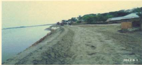
Fig: Pre-work Condition of the road
