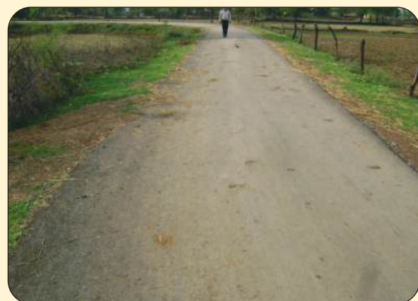
Initiation of distress at JGT laid section after 26 Months (2009)
