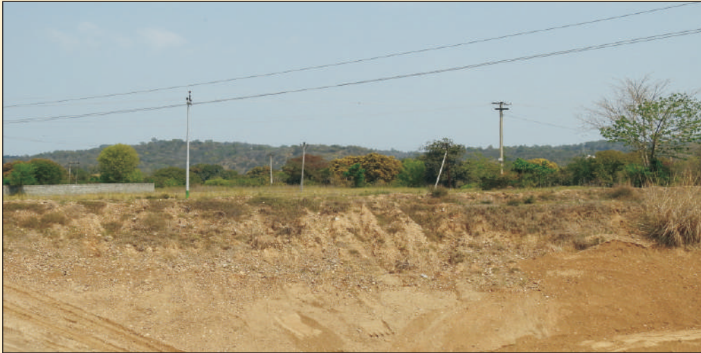
Destabilized hill slope
