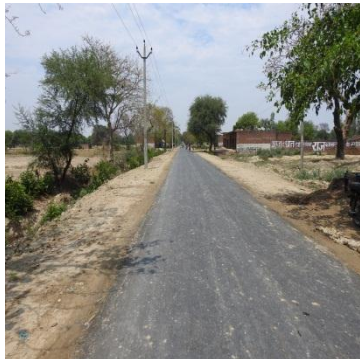
Condition of Road after 3 years
