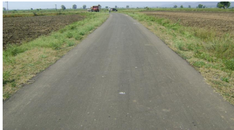
CONDITION OF ROAD AFTER 4 YRS.
