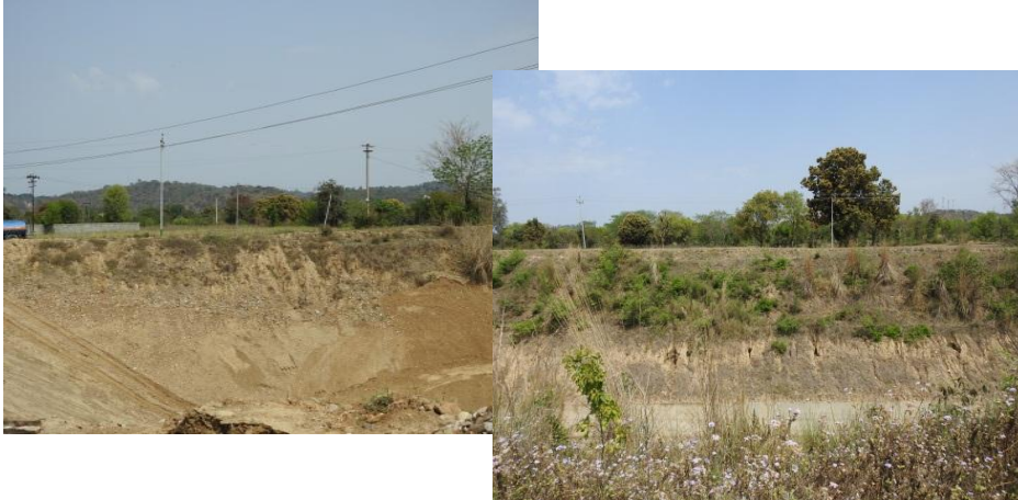
Eroded Slope of Cuttings
