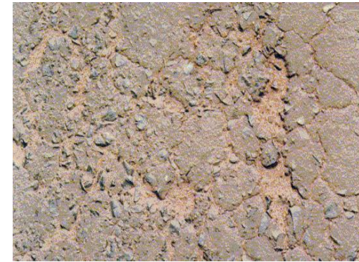
Potholes on surface
