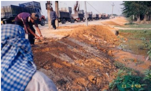
Eroded slope of road embankment
