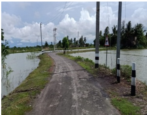
CONDITION OF THE ROAD EVEN AFTER ELAPSE OF 3 YEARS
