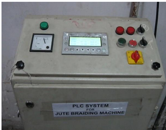
Fig.6.2.5. Control panel for jute braiding machine
