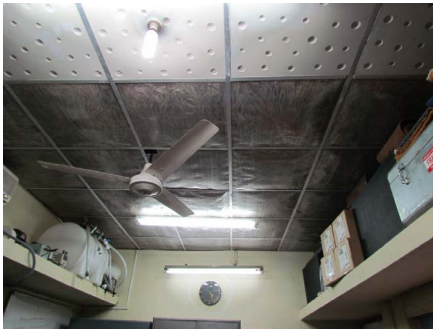
Figure 51: Acoustics laboratory, Mechanical Department, IIT Kharagpur Mineral Fiber Board Ceiling Replaced by Jute Acoustical Ceiling.
