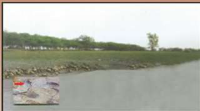
CONDITION OF JGT TREATED RIVER BANK AFTER 23 YEARS
