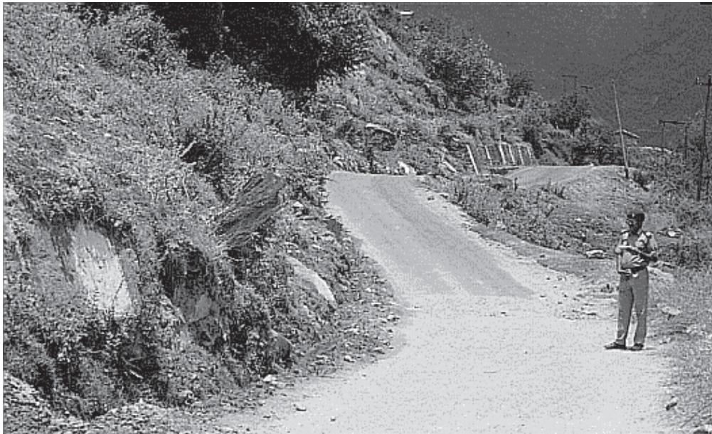
Fig. 4 Road sinking has stopped towards Joshimath side (Monitored after one year)
