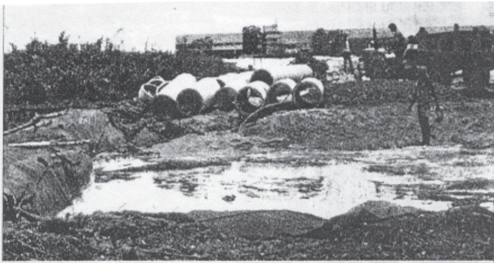
Fig. 10 Jute geotextiles were laid in the creek portion and sand filling in the process.
