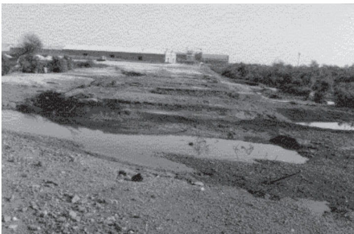
Fig. 13 The untreated stretch of embankment completely damaged by the cyclone of 1996.
