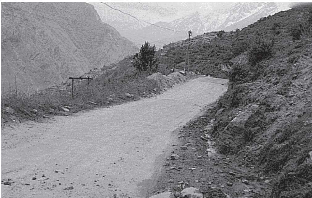
Fig. 5 Road stretch towards Manali side has become stable (monitored after one yer)
