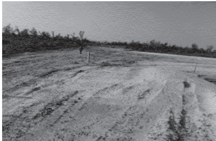
Fig. 12 Monitoring after the cyclone of 1996 shows the embankment stretch treated by jute geotextiles is not damaged.
